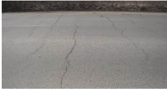
Figure 2.10: Traditional Transverse Cracking of Asphalt Pavement
