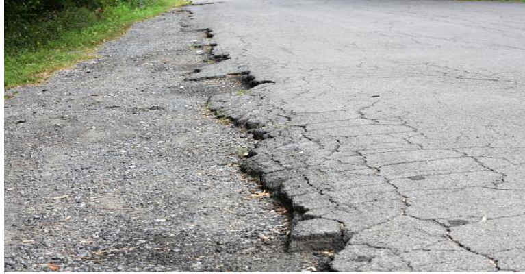
Figure 2.5: Edge Cracking of Asphalt Pavement
