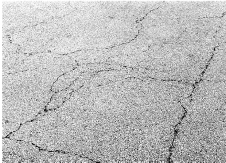
Figure 2.4: Block Cracking of Asphalt Pavement
