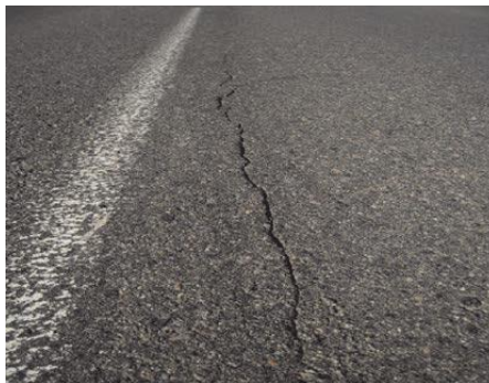
Figure 2.6: Longitudinal Cracking of Asphalt Pavement
