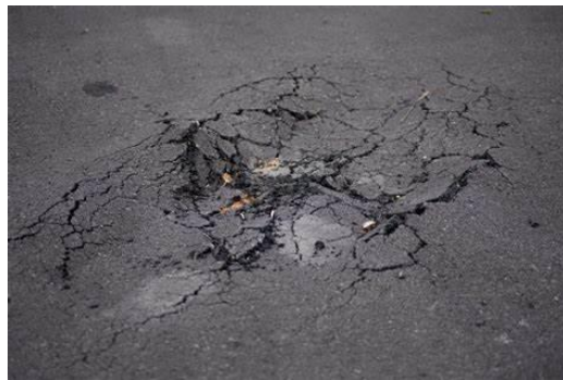
Figure 2.9: Moisture Damage of Asphalt Pavement
