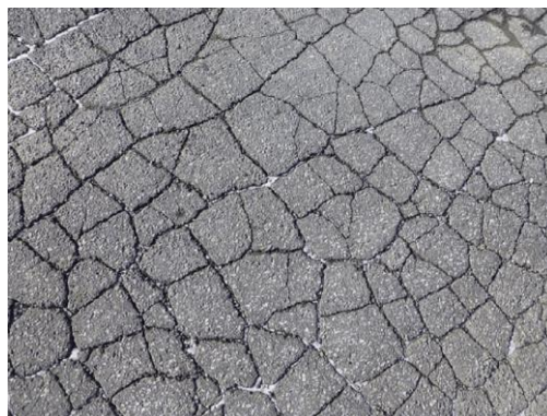
Figure 2.8: Alligator Cracking of Asphalt Pavement
