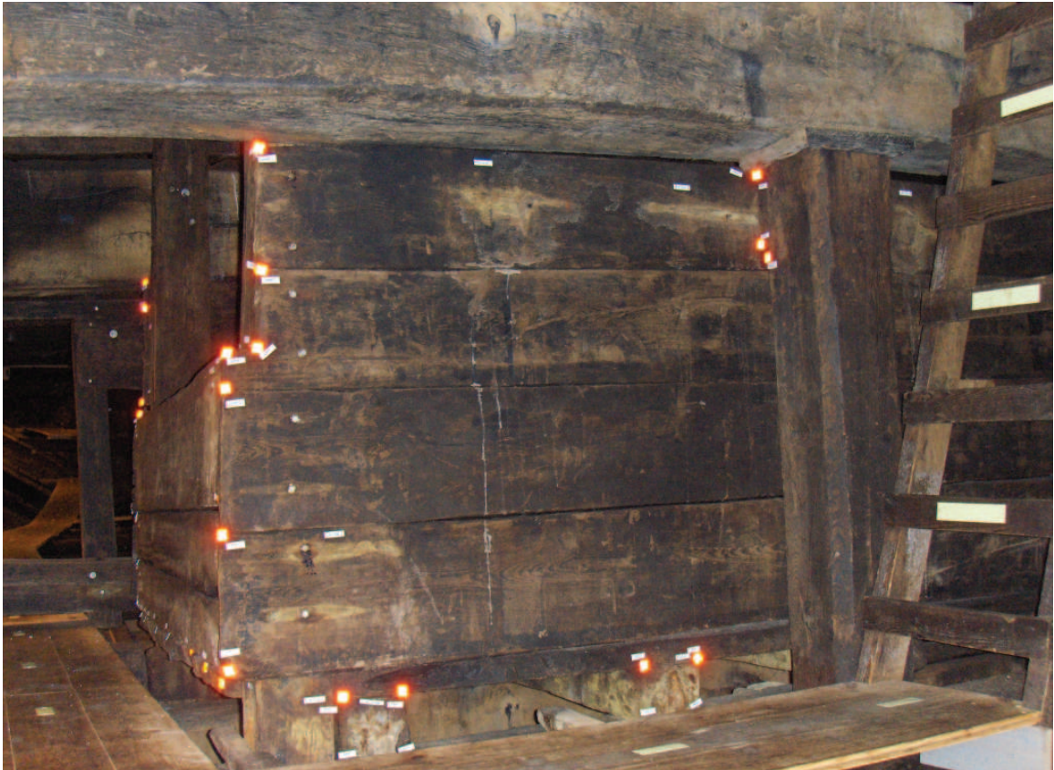
Figure 4-5: The jog in the starboard side of the forward wall. It is outlined by the bright reflective tape along the forward edge. The shorter side wall of the galley can be seen in the left side of the photograph.
