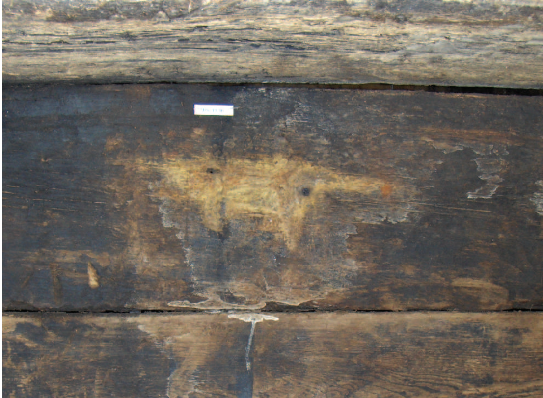
Figure 4-13: Stains left in the wood from iron corrosion products. Such stains leave evidence of fasteners and artifacts.
