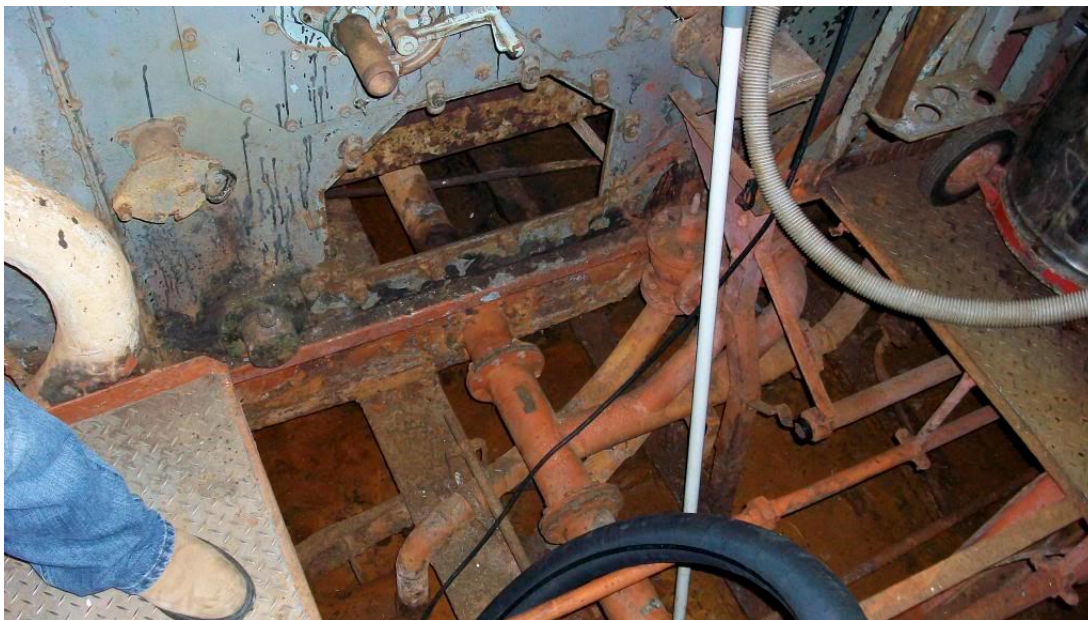
Photograph 59: Laffey 's hull beneath forward boiler. The corrosion is most visible at upper center, through removed access hatch.
