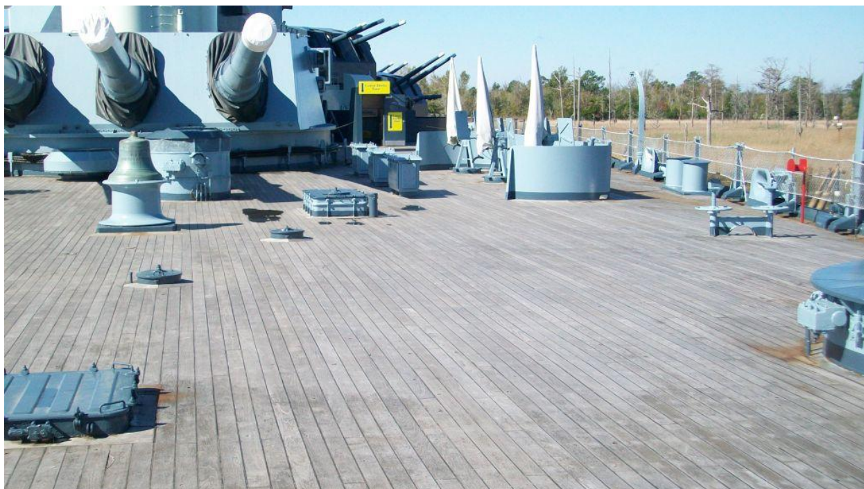
Photograph 20: North Carolina's restored teak deck, viewed abaft Turret #3. The tour route access hatchway is visible adjacent to Turret #3.
