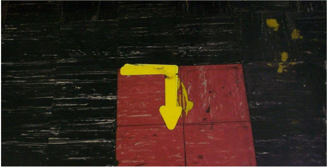
Photograph 44: Most of Yorktown 's wayfinding arrows are small, and some need replacing.
