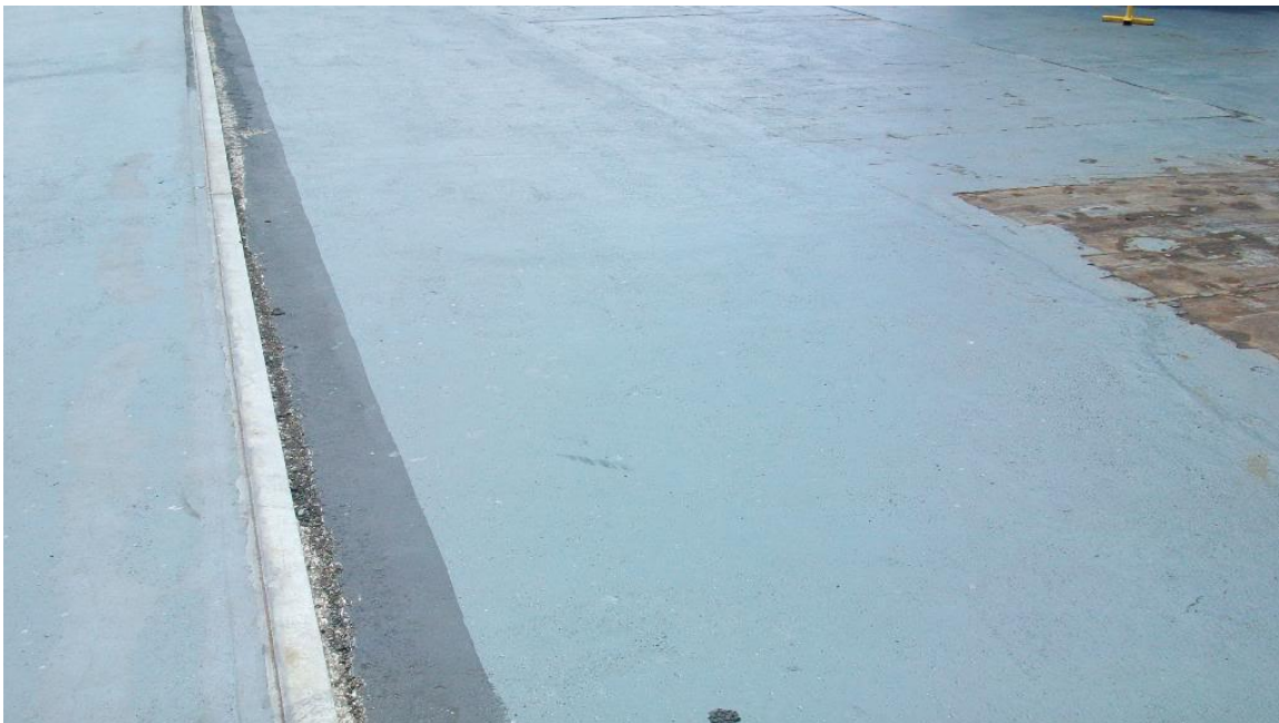
Photograph 84: Portion of asphalt compound test section. Wood stripped of the rubber coating is visible at right.
