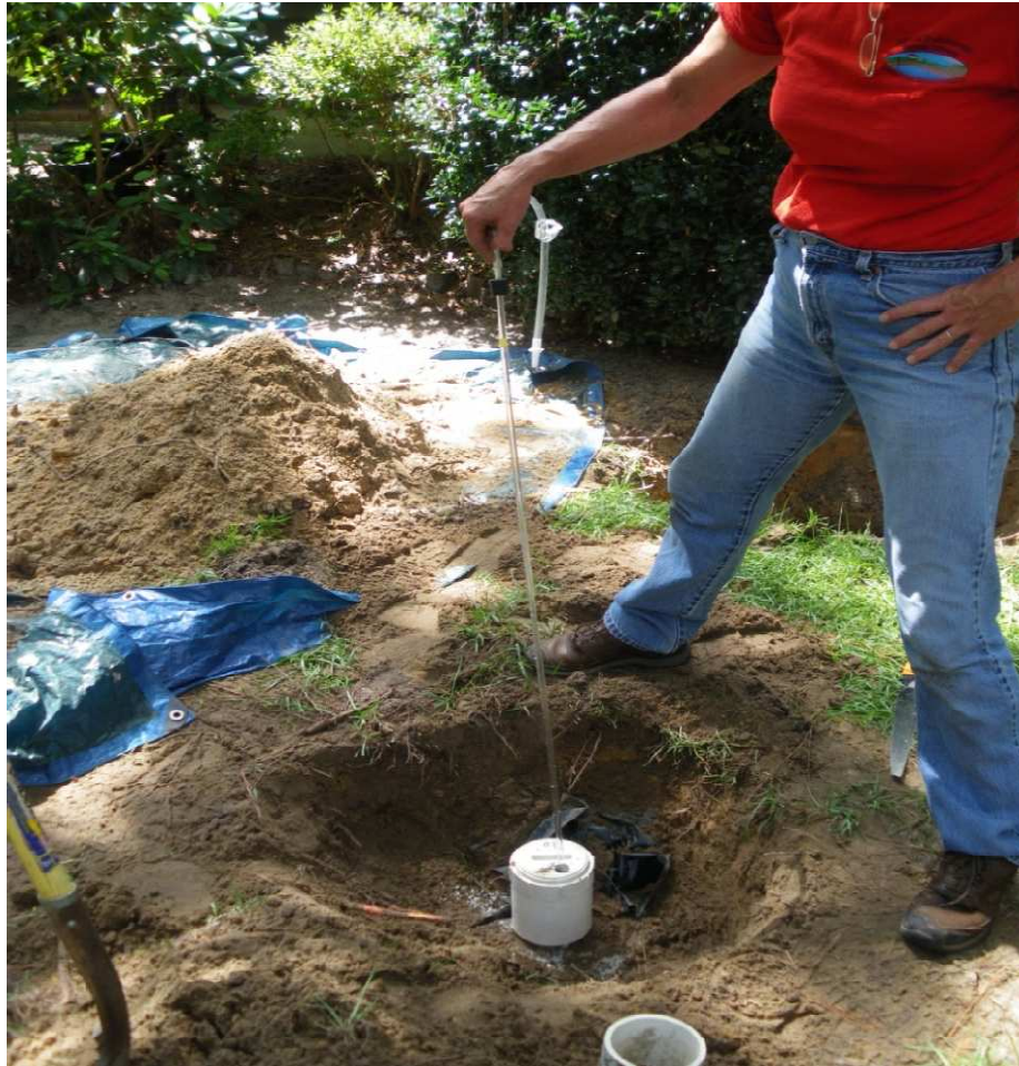
Figure 4. Installation of the PVC Cleanout at Site 2. Flex tubing was attached to the rigid tubing and fitted with a nipple used for connection to the peristaltic pump, which was used to retrieve effluent samples from the inner and outer section of the OWTS.
