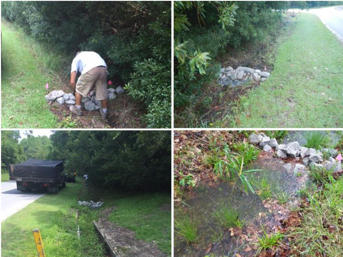
Figure 14. Installation of rock check dams in drainage swale along Croatan Forest Road, near the Cedar Point Campground. Check dams reduce runoff velocity and allow temporary ponding of water behind them, encouraging infiltration and pollutant treatment (bottom-right).
