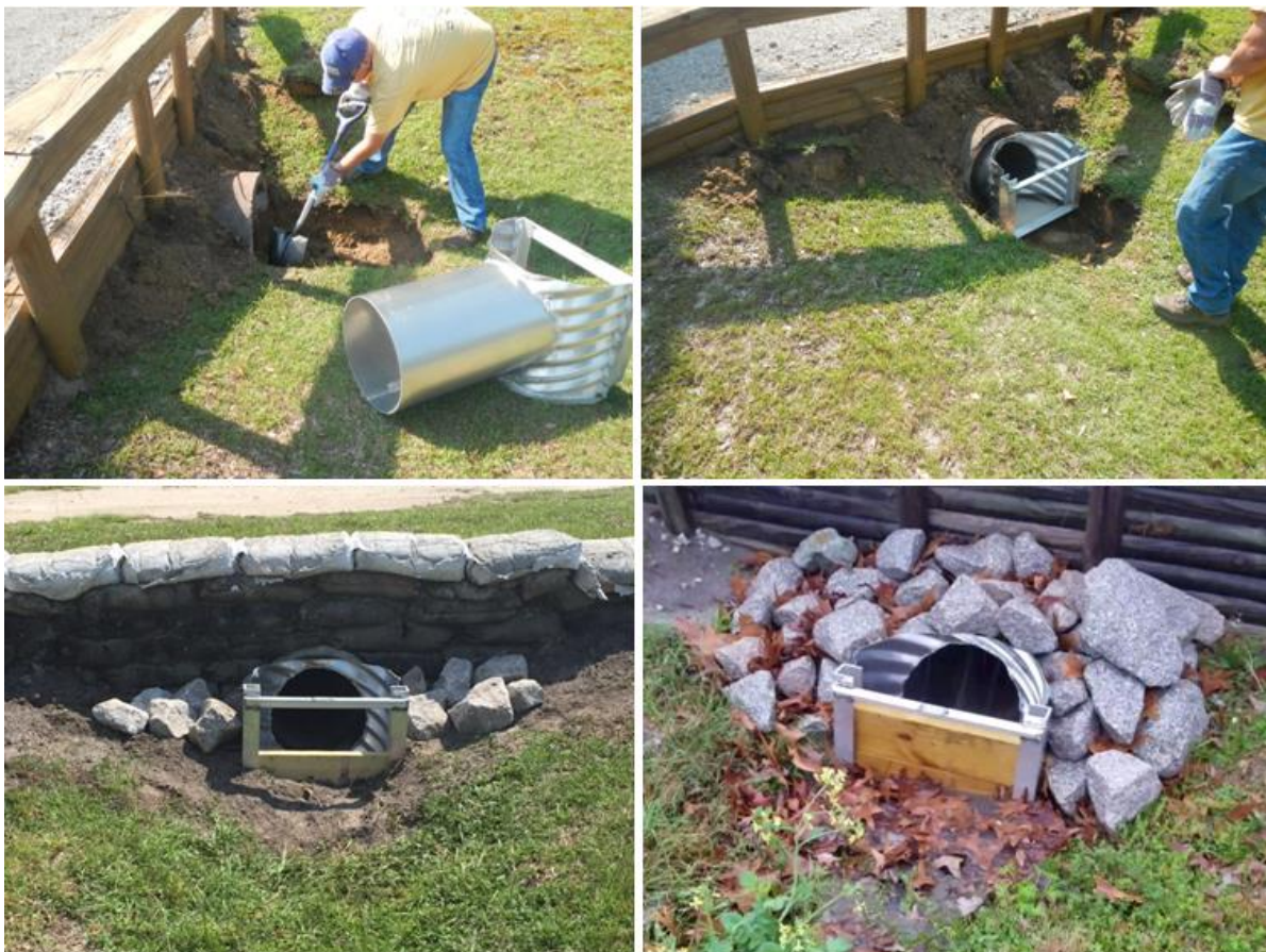
Figure 10. Installation of water control structures in Ocean Spray drainage culverts. Soil around the culvert was removed to allow placement of the structure. Wooden boards were placed within the frame in order to reduce velocity and volume of runoff discharging from the swale (bottom-right).
