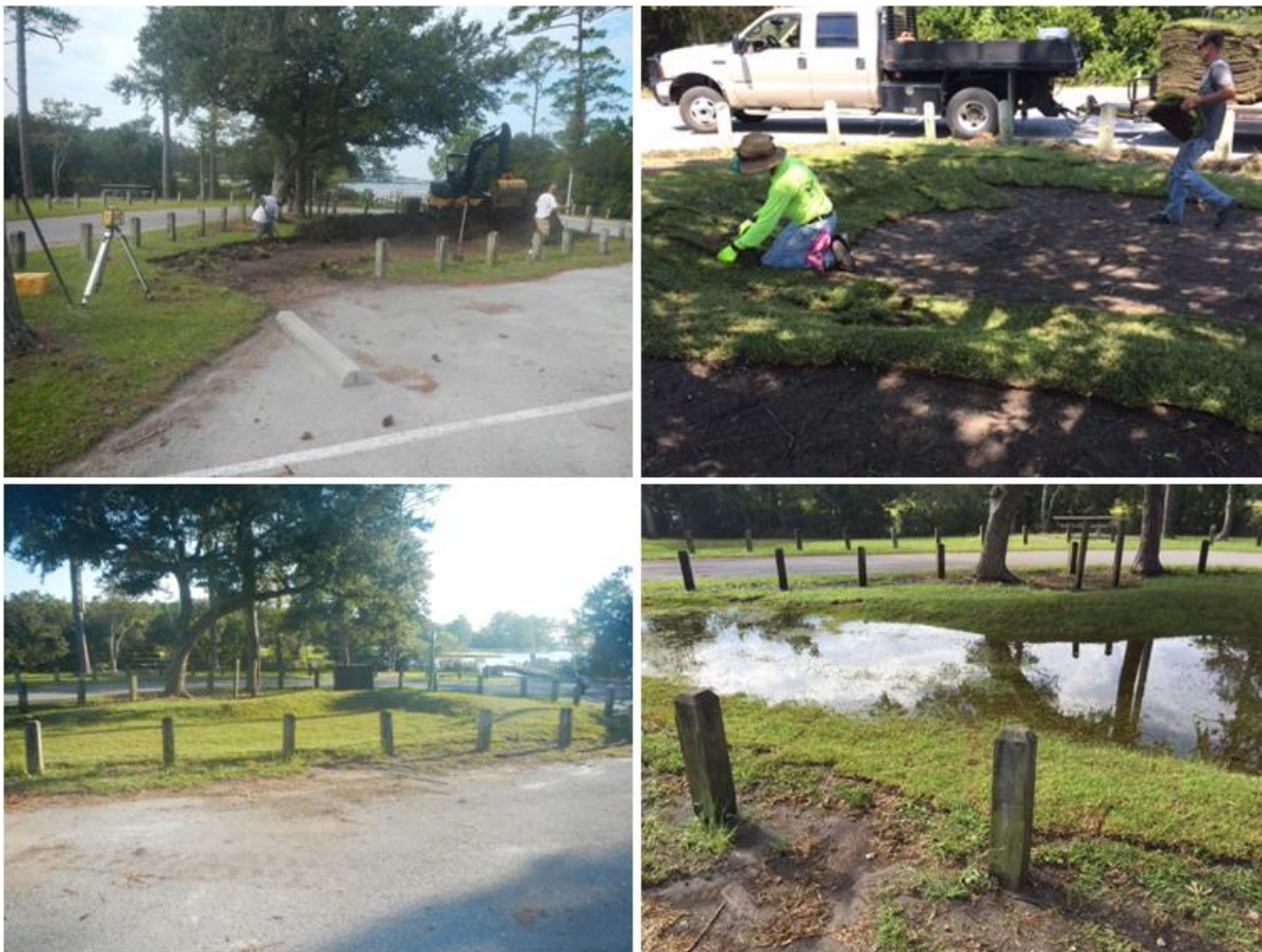
Figure 18. Rain garden construction at the Cedar Point Tideland Trailhead parking area and boat ramp. Rain garden is shown storing runoff from a storm shortly after installation (bottom-right).
