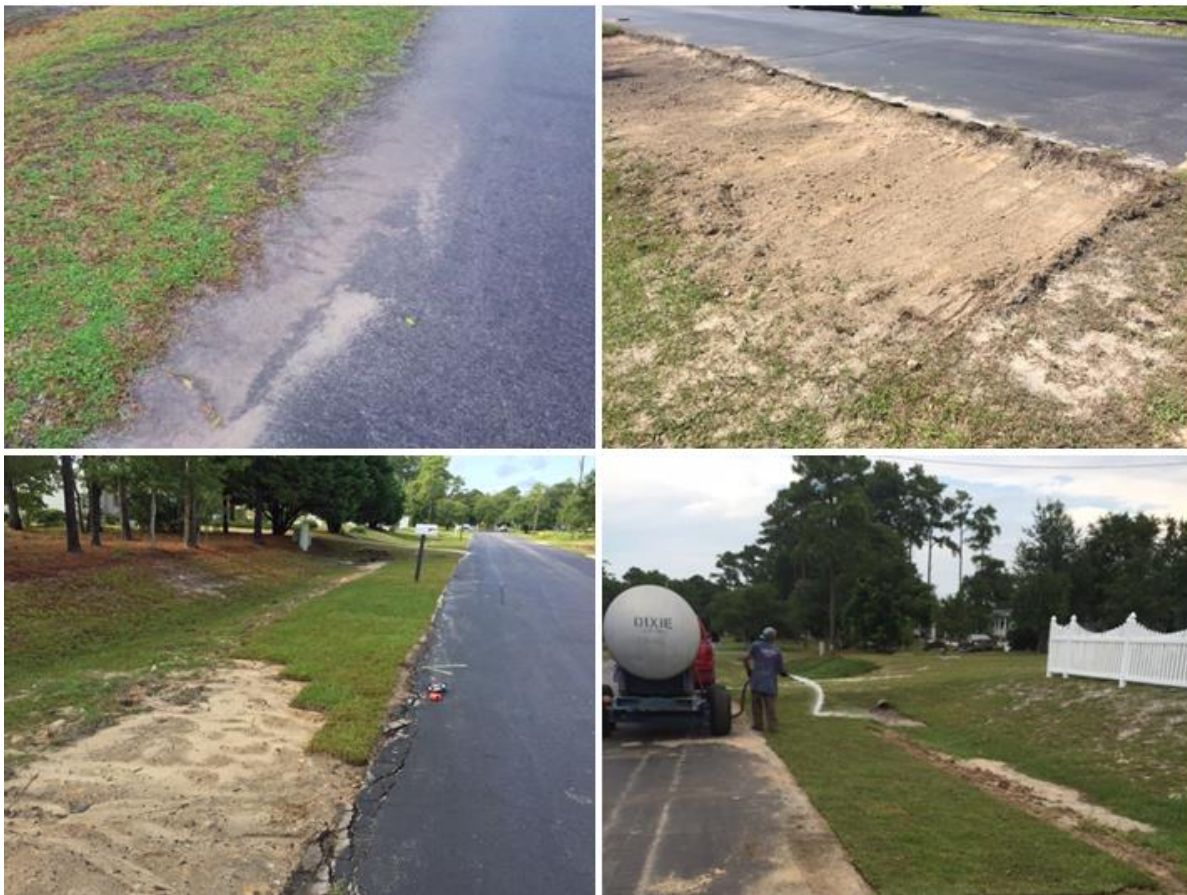
Figure 12. Swale stabilization and enhancement process in the Ocean Spray community. Grass and soil along the edge of the road was excavated, graded, resodded, and watered, allowing runoff to enter swales more effectively and promoting infiltration.
