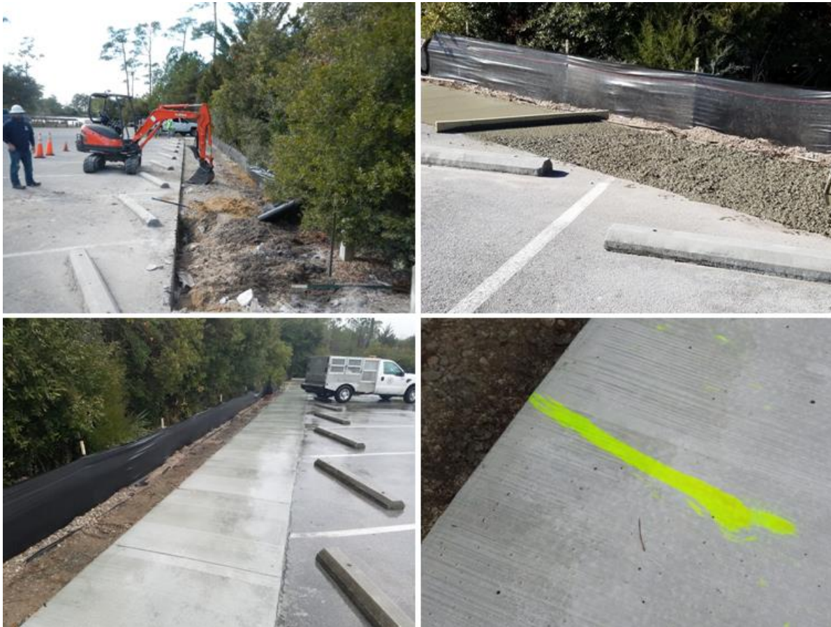
Figure 16. Construction of the new walkway at the Cedar Point Tideland Trailhead parking area and boat ramp. Walkway edge was made level with parking lot and graded to divert runoff toward forested area for infiltration, as shown by the tracer dye (bottom-right).
