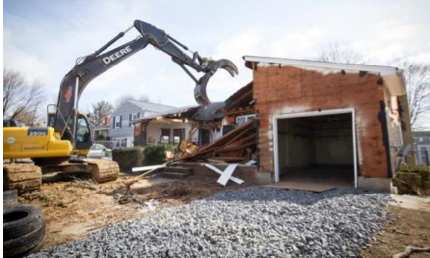
Figure 3.6: Example of a house bought and torn down by local government (Buyout). Source: FEMA 2018c
