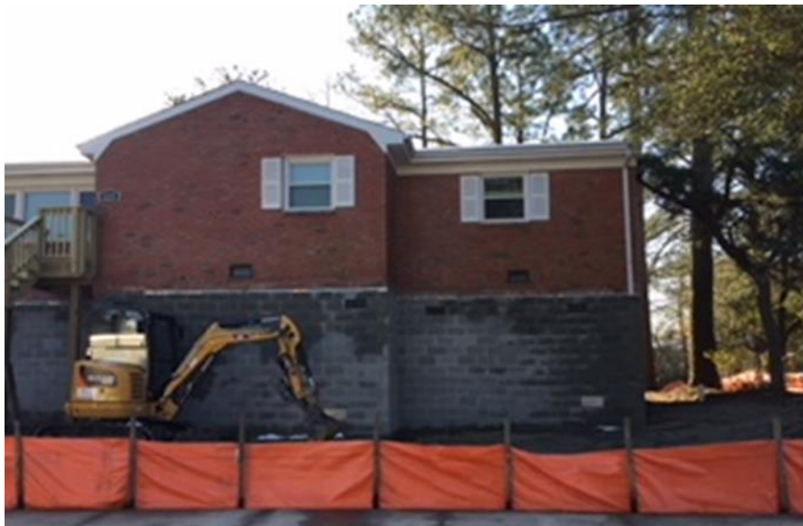
Figure 3.7: Example of a house being elevated above ground (House elevation program). Source: Courtesy Jamie Kruse
