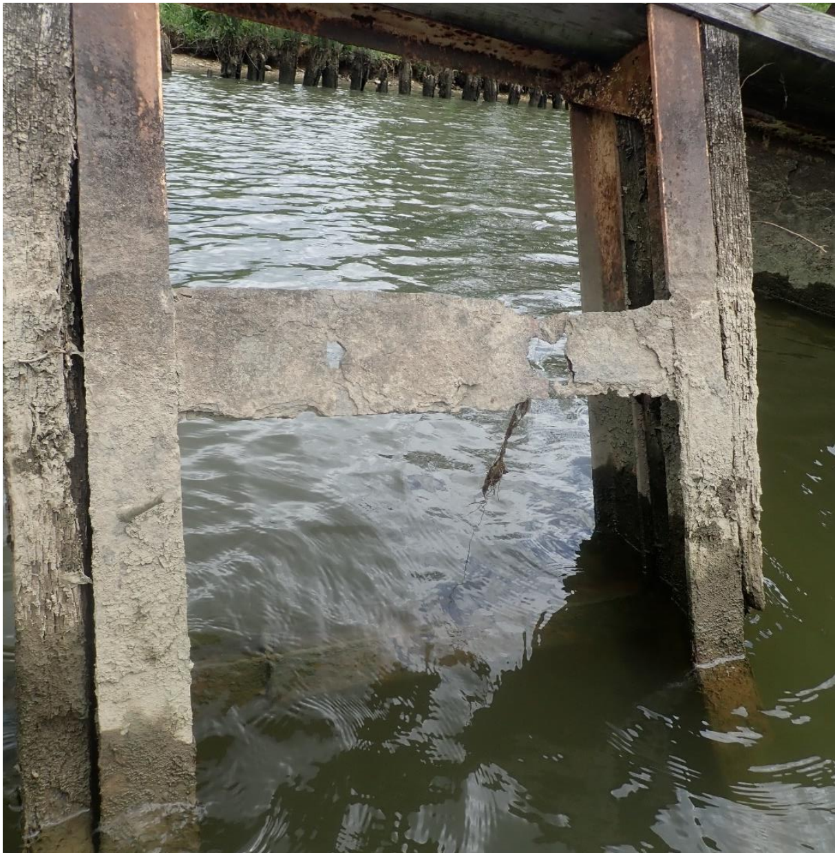
FIGURE 6.28 Metal cross bar showing extensive rust and formation of holes (Photo Credit: Nathan Richards, 2021).
