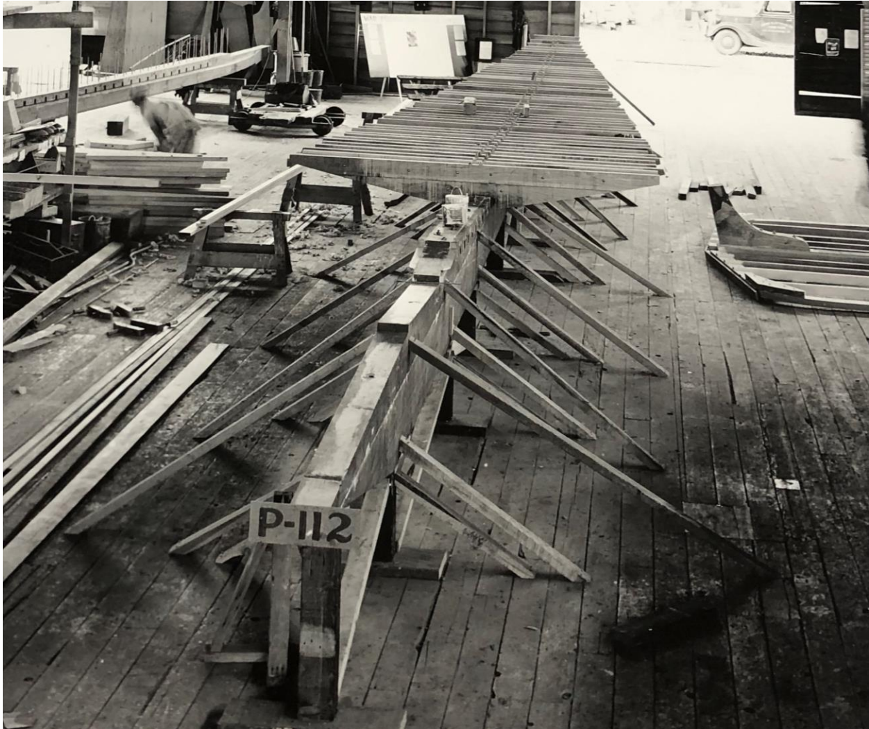
FIGURE 6.1 Construction of P-112, a 104' ARB Design 235A, at Stephen Bros. Ship Building Company, show a process that is consistent with construction of wooden vessels (Photo courtesy of Haggin Museum, 1942).
