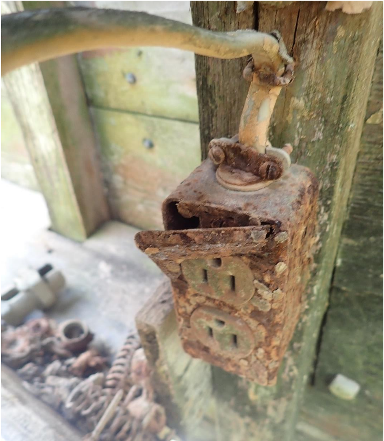
FIGURE 6.14 NEMA 5-15 AC electrical socket mounted to a hanging knee in the engine room of the Sea Scout Wreck (Photo Credit: Nathan Richards, 2021).
