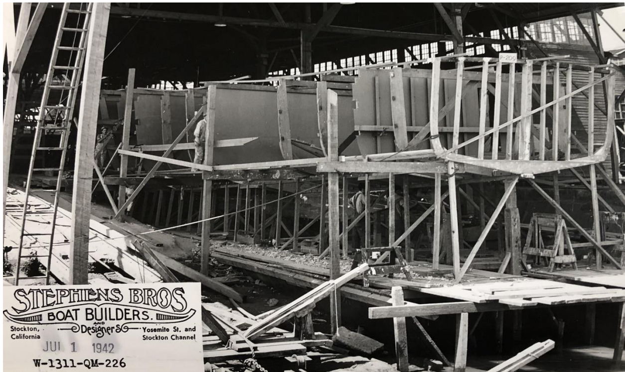
FIGURE 5.3 Photograph of bulkheads being installed on a 104' ARB (Probably a Design 235A based on the thin keel in the aft section) (Photo courtesy of Haggin Museum, 1942).
