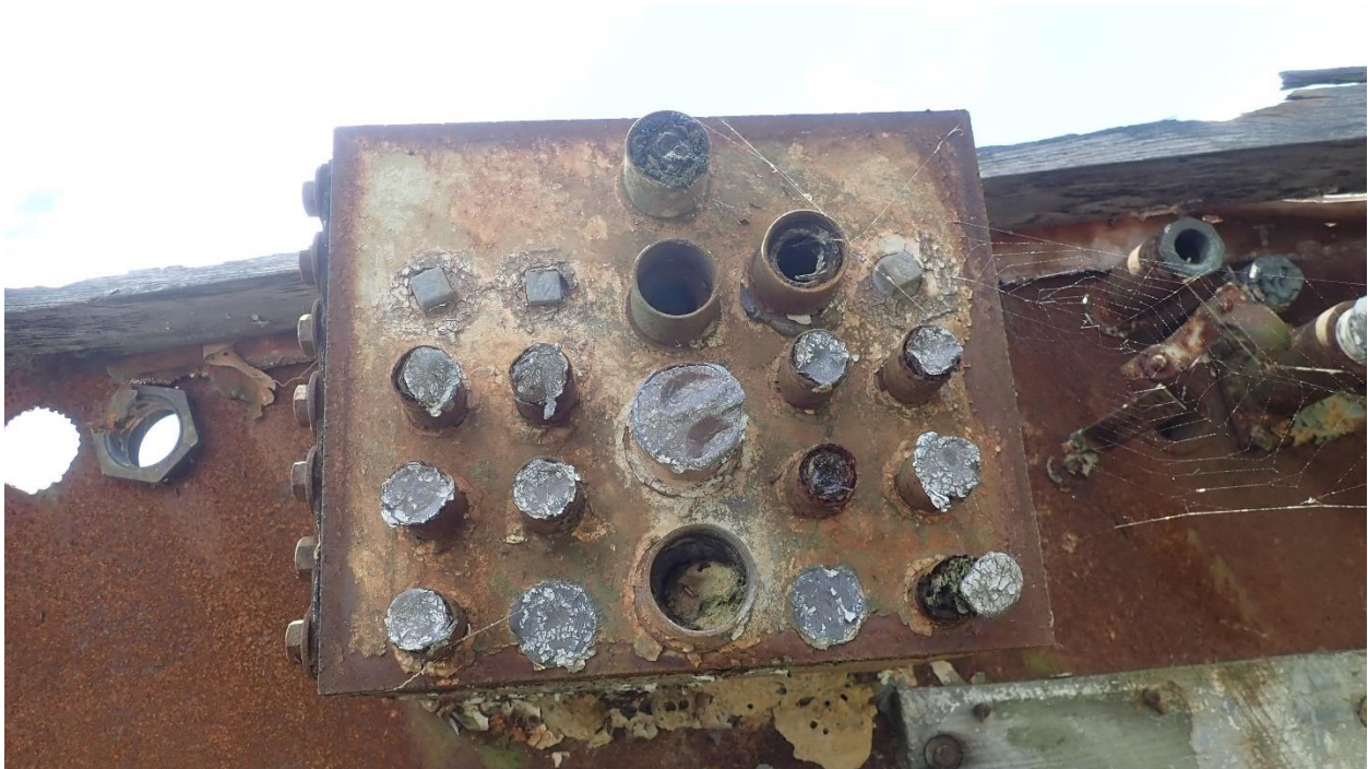
FIGURE 6.11 Original electrical paths in Bulkhead 6 of the Sea Scout Wreck that are capped or fitted with PVC pipes (Facing south) (Photo Credit: Nathan Richards, 2021).
