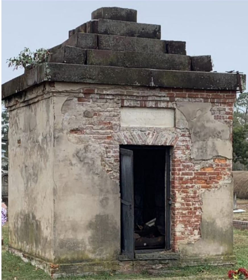
Figure 1.01: The east wall of the Rhem Vault. Virginia creeper can be seen growing through the roof on the left, and additional roof supports are visible on the right corner of the roof. Photo by Dr. Megan Perry.
