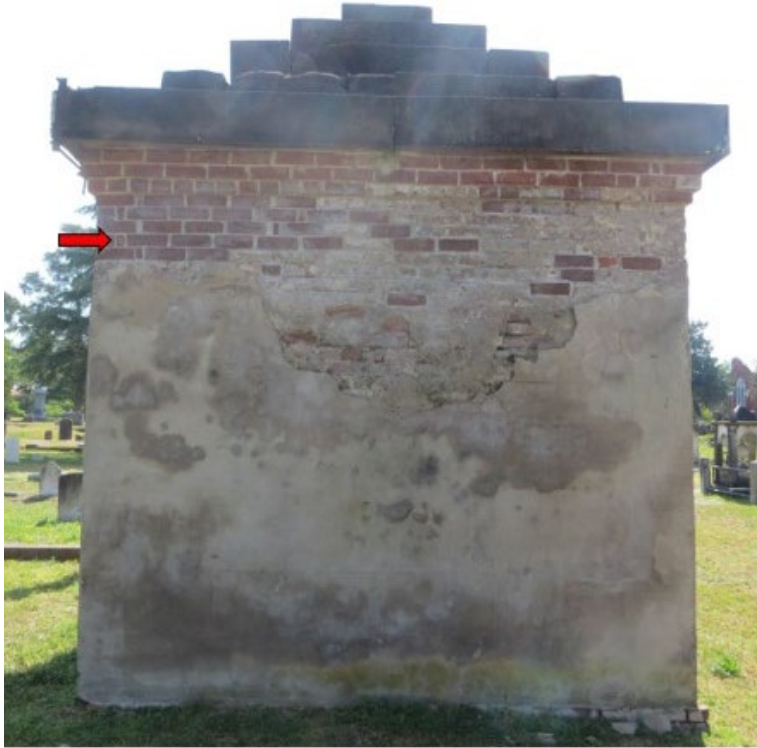
Figure 4.02: The exposed brick on the Western wall shows two stretcher courses and one header course on the roof with a partial Rat Trap bond. The partial Rat trap bond is marked with a red arrow. Photo by Jalyynn Stewart.
