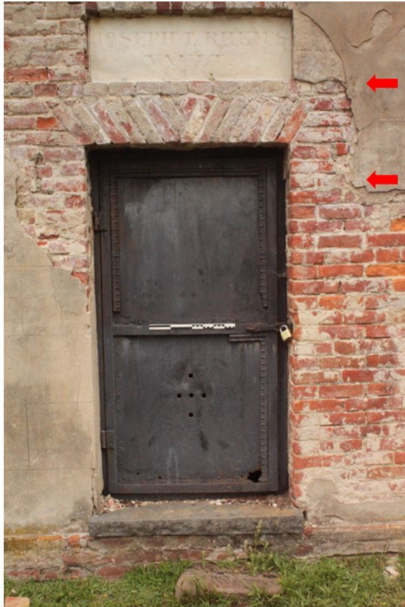
Figure 4.01: The exposed brick on the eastern wall of the Rhem Vault shows a common bond brick pattern with a header course every 5 th or 6 th course. Header courses are marked with red arrows. Photo by Jalyann Stewart.
