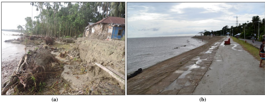
Fig. 6 Evidence of riverbank erosion (a); and the revetment in Ramgati (b)
