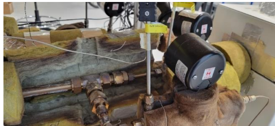
Figure 109: HEX1 hot line entrance and cooling line exit union insulation
