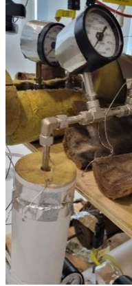
Figure 110: HEX1 hot fluid exit line exposed for inspection.
