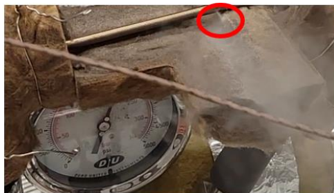
Figure 115: Pin hole venting steam shown circled in red.
