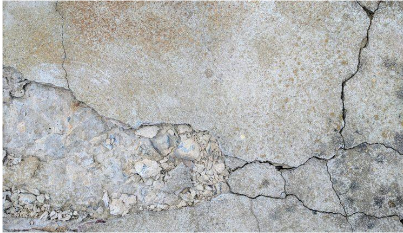
Figure 1. Structural deterioration due to concrete cracking and spalling
