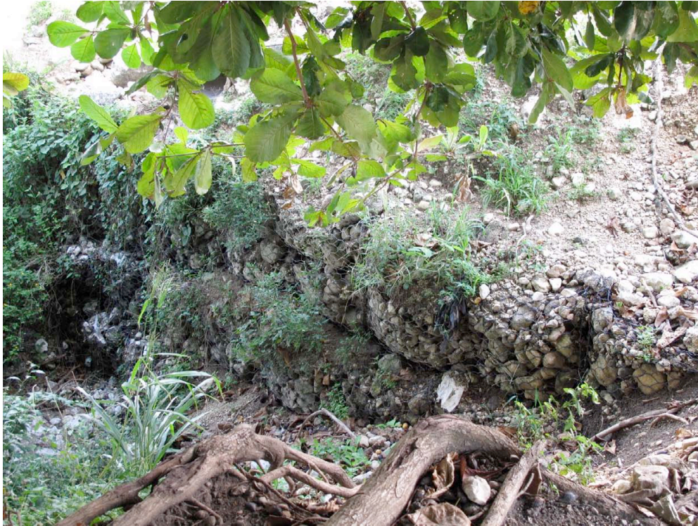
FIGURE 59. Rock clusters used for the road to Savannah-la-Mar. These rock clusters were found along the shore throughout Survey X. They were artificially placed here to raise the historic road of Savannah-la-Mar beyond the reach of storm surge and wave action. (Photo by, author October 11, 2009.)
