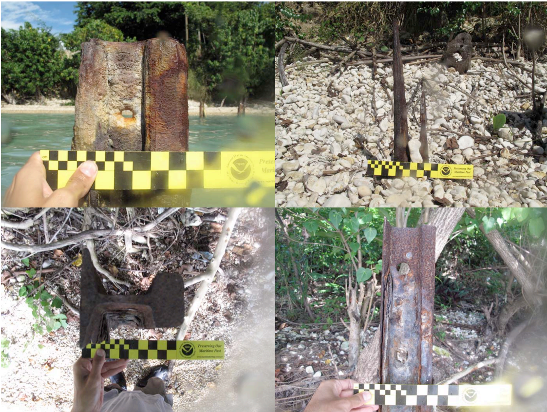
FIGURES 55, top left , 56, top right , 57, bottom right , and 58, bottom left . Photos showing the I-beam’s designed width, an example with severe deterioration, designed holes, and their distinctive I-beam shape, respectively. (Photos by author, October 25, 2009.)
