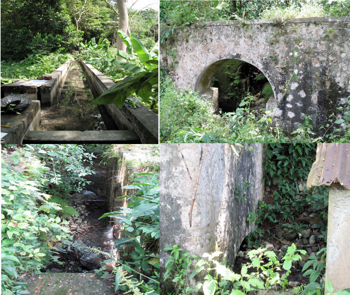
FIGURES 78 top left , 79 top right , 80 bottom right , and 81 bottom left . Photographs of the Coldeer Shaftson Aqueduct from the south, Waterwheel Structure from the west, water leaving the Waterwheel Structure from the south, and water falling into the Waterwheel Structure from the north, respectively. (Photos by author, 2009.)
