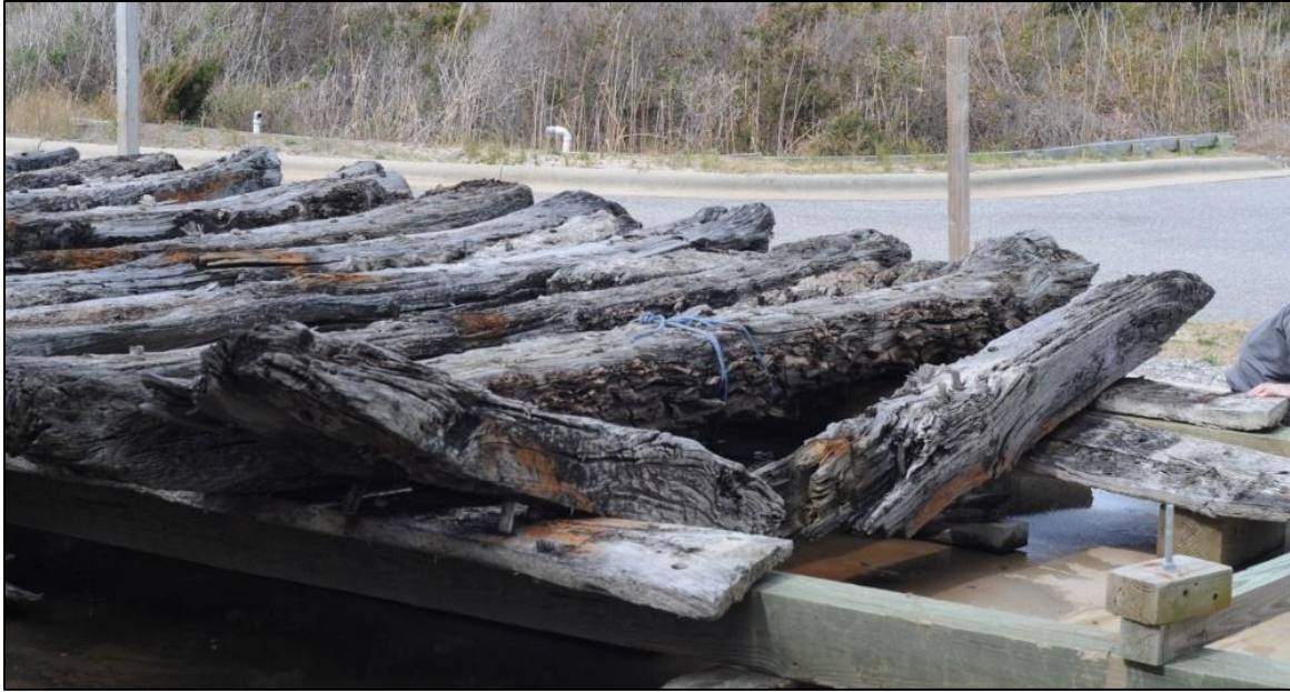
FIGURE 133. Entire frames have collapsed and continue to disintegrate without any protection from the elements. (Photo by Author, 2012)
