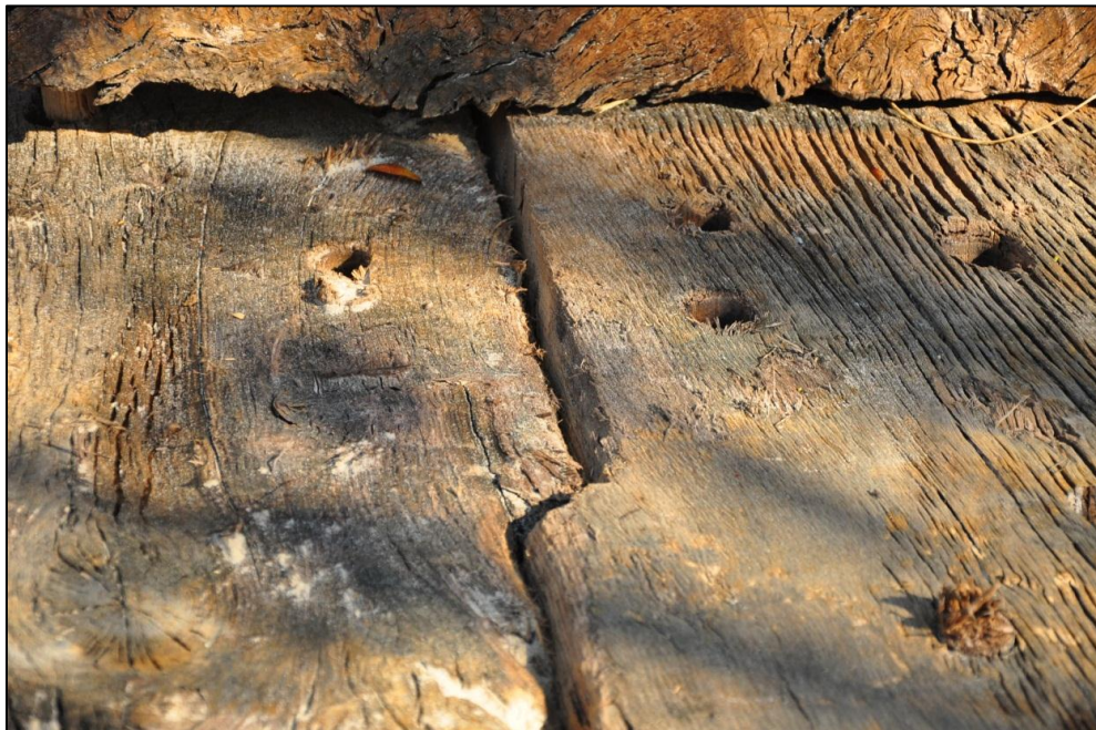
FIGURE 146. A joggled plank seam, 1 day after removal, April 2010. (Courtesy UAB)
