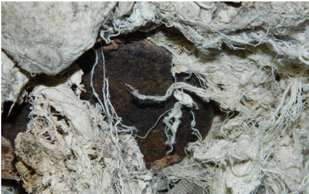
FIGURE 31. Corroded metal rod inside the support beam (Author 2013)
