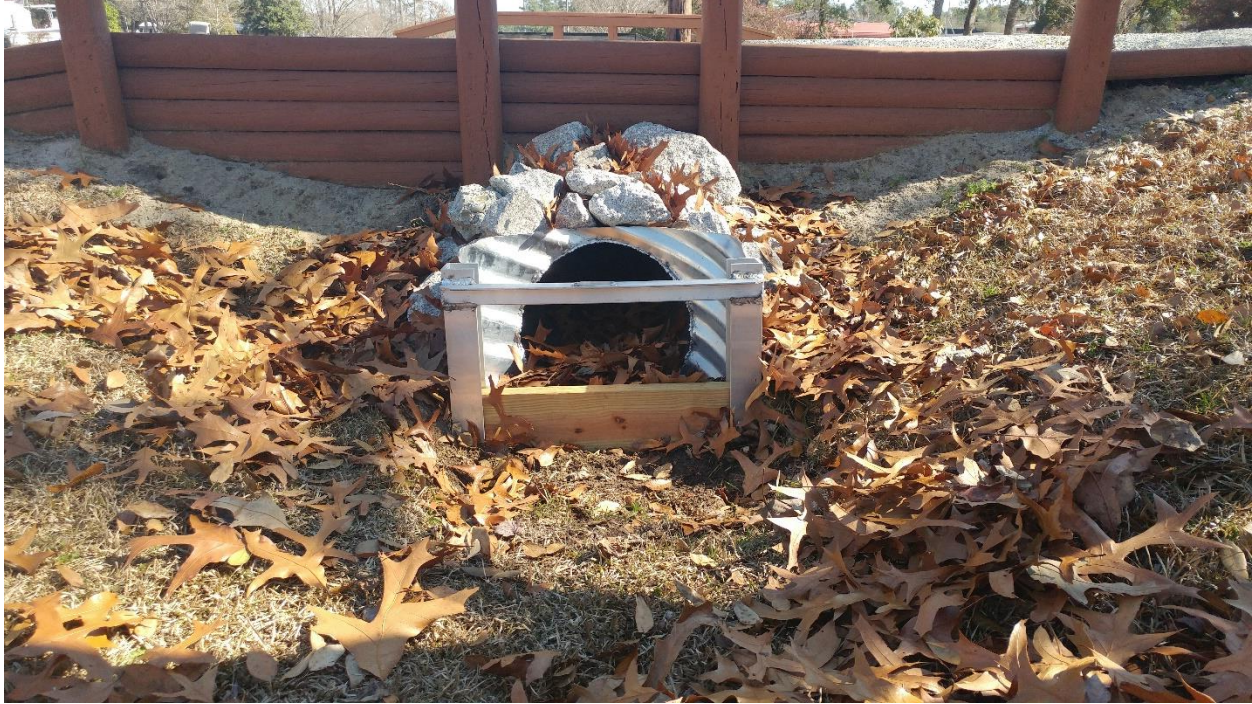
Figure 10: Water Control Structure installed
