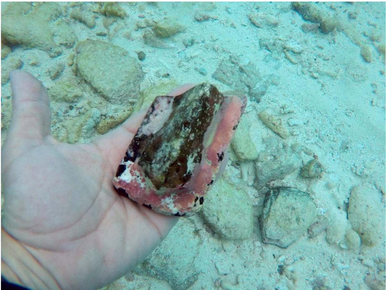
FIGURE 4.8. Partial deck prism observed during 2017 post-hurricane condition assessment. (Image from NPS, 2017).
