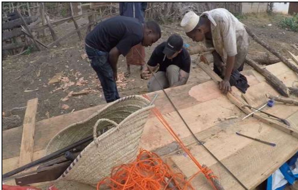
Figure 30: Author forms rebar guide for Y-frames and checks arm angle with handi under supervision of Mfundu Muddi, Tongoni Village, Tanga Region (Photograph by Madeline Roth)
