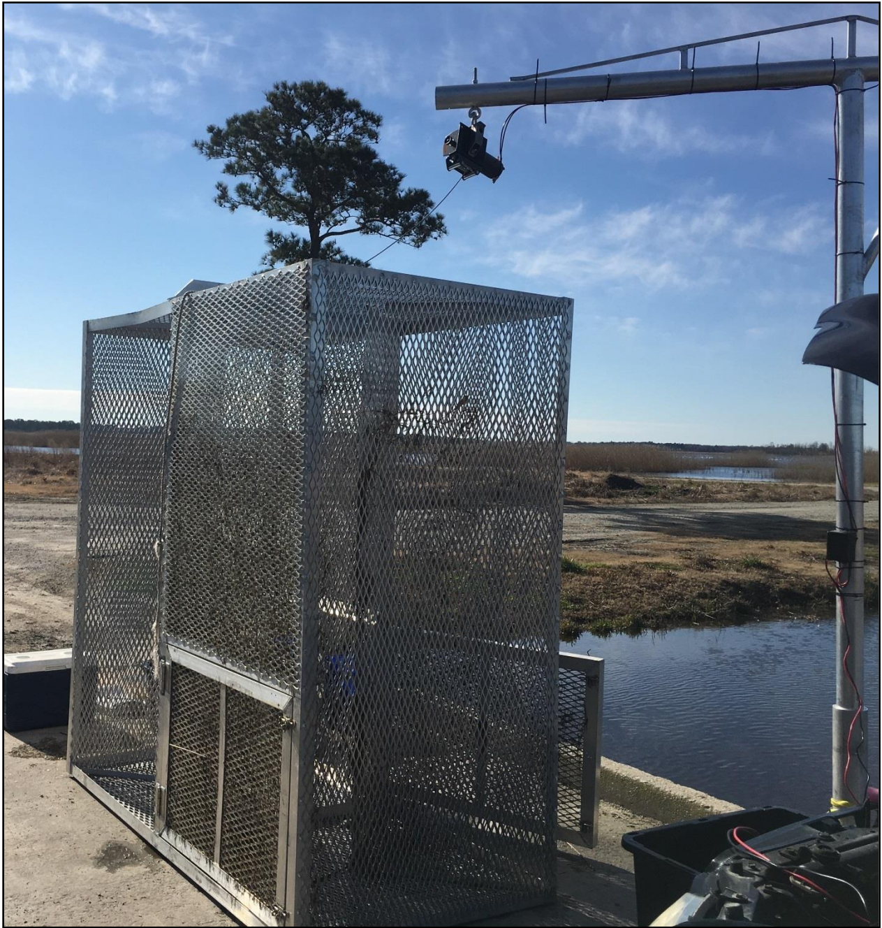
Figure 3.6. Lift system, electric winch, and custom-built dual-sided fish trap deployed in the top-hinged gate during the 2016 sampling period at Waupoppin Water Control Structure, Lake Mattamuskeet, North Carolina.
