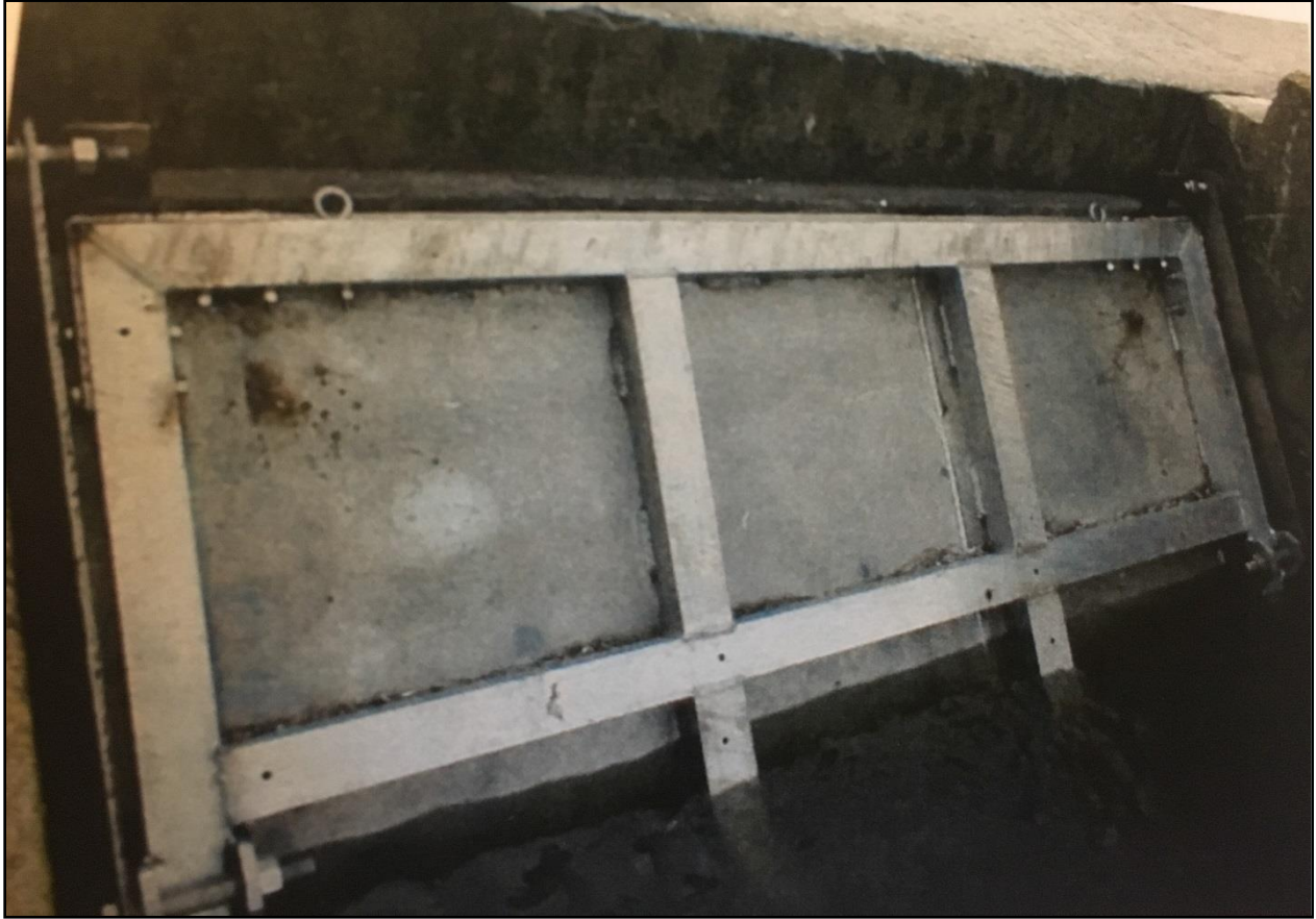
Figure 3.4. Photograph of one of the current top-hinged flapgates in place at Waupoppin Water Control Structure, Lake Mattamuskeet, North Carolina. Godwin (2004).
