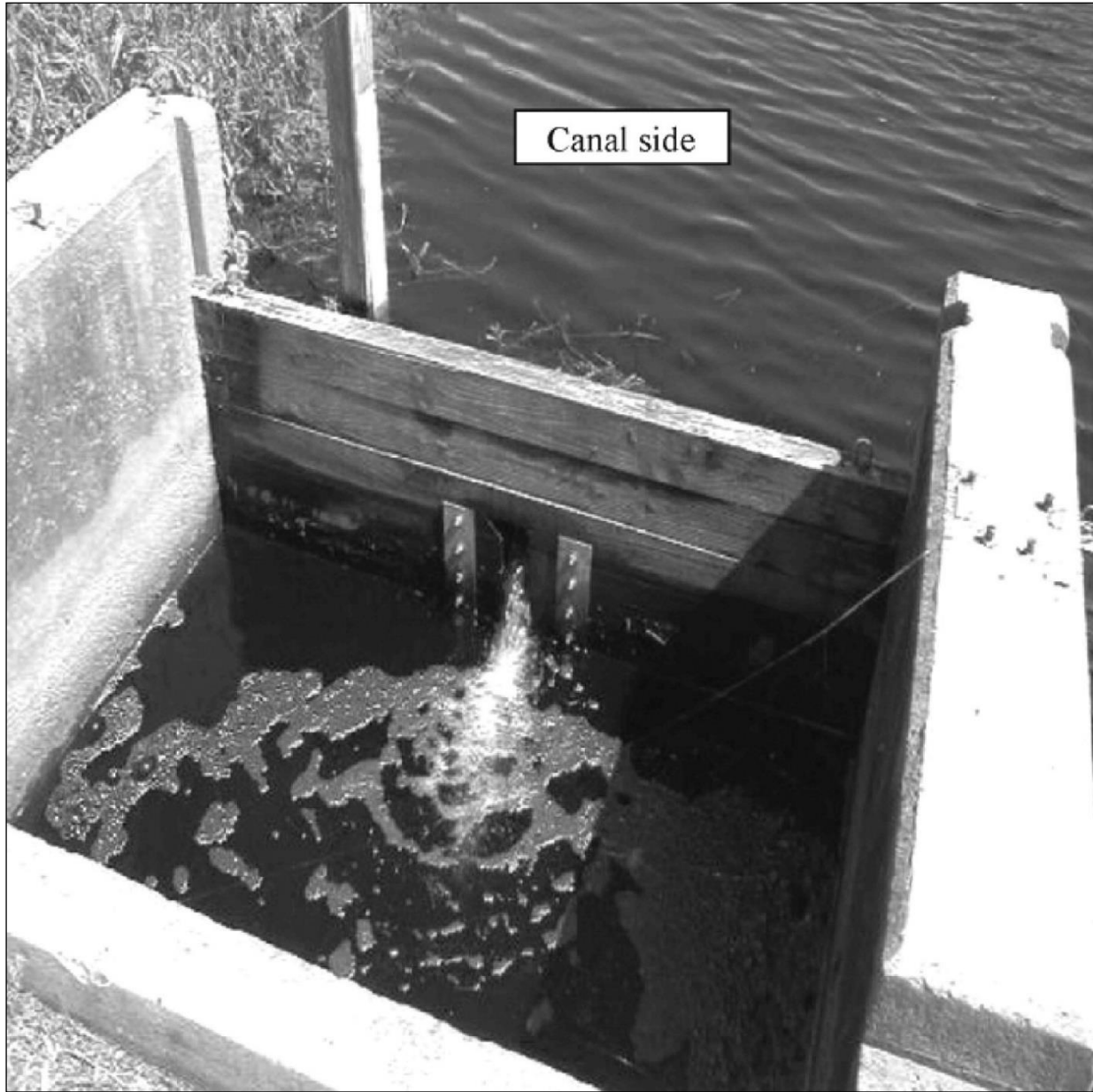
Figure 3.3. Photograph of one of the fish passage slotted weirs that were installed in 1996 in existing wooden stop blocks to enhance fish and blue crab passage, Lake Mattamuskeet, North Carolina. Rulifson and Wall (2006).
