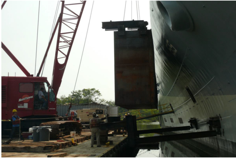
Figure 32. Image showing the portable cofferdam being fitted to hull of USS North Carolina (Image from Ocean Technical Services LLC.)
