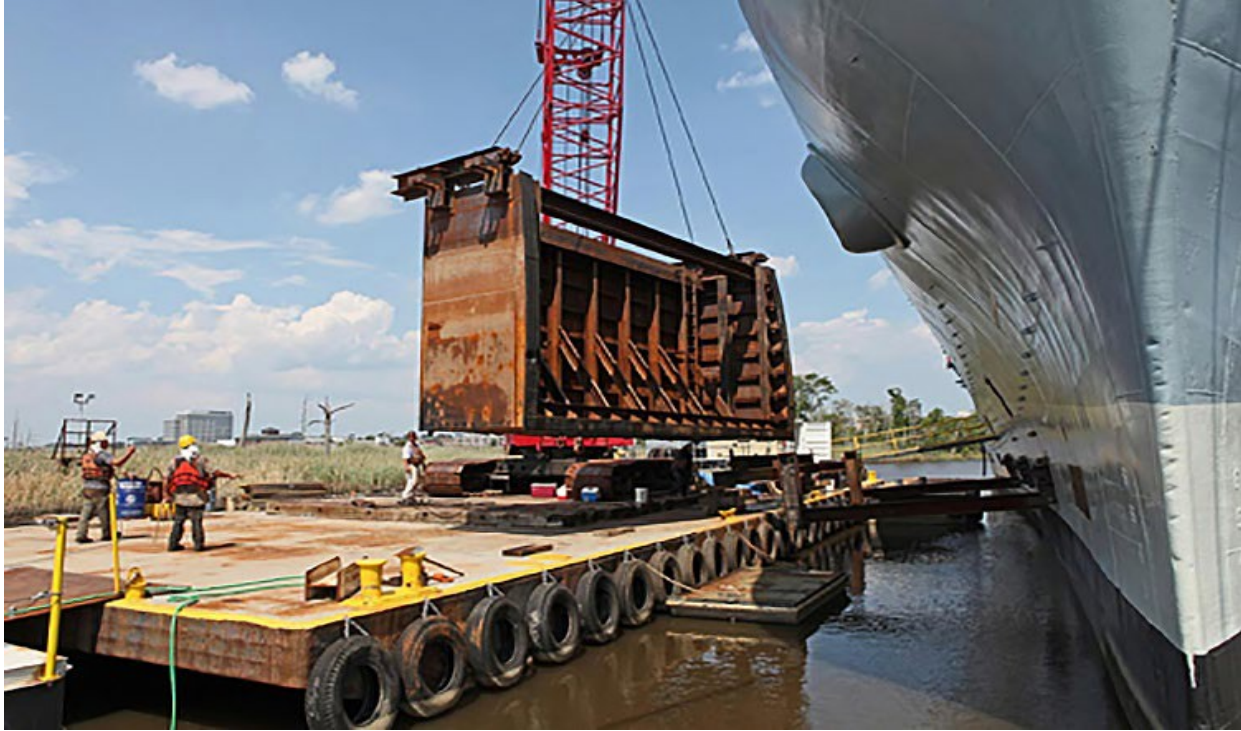
Figure 6. Portable Cofferdam being fitted to USS North Carolina during 2011 starboard bow repairs. Photo from http://www.jmsnet.com/projects/battleship-uss-north-carolina/
