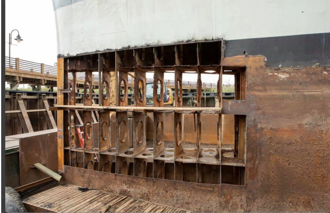
Figure 40. Port side view of current hull repairs along the bow. (Image by Joe Hollifield 2020)
