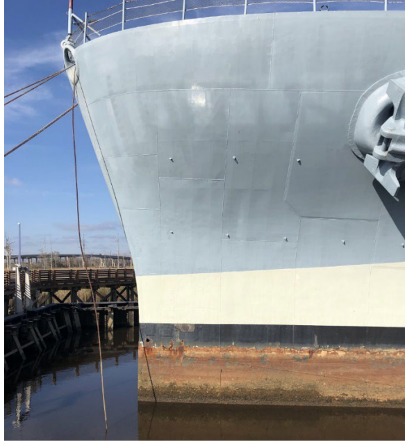
Figure 38. Image showing corrosion along the wind/waterline with a hole near the stem of the ship. (Image by Author 2020)
