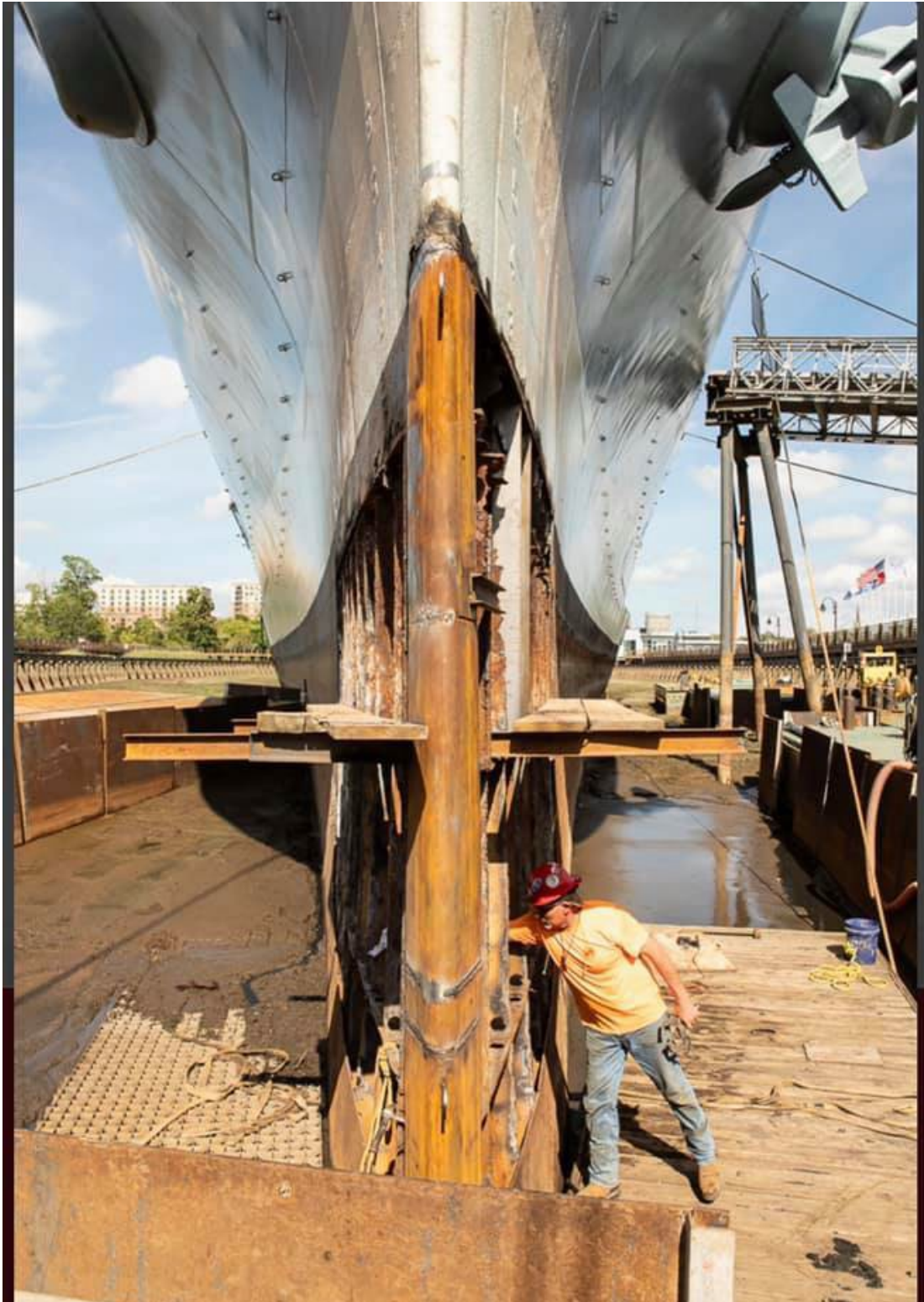
Figure 41. Front view of bow showing current hull replacement progress. (Image by Joe Hollifield 2020)
