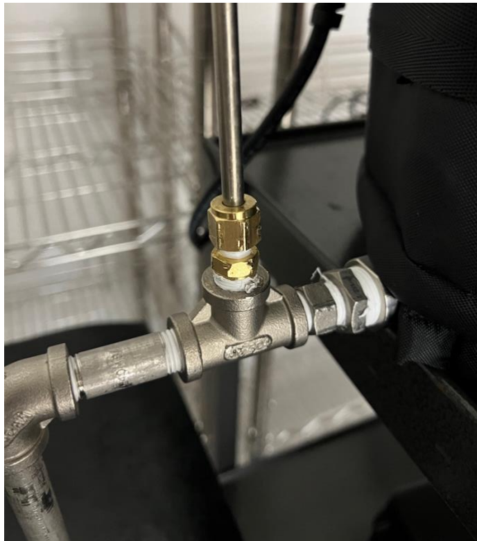
Figure 20: Thermocouple compression fitting and the tee connector in the experiment
