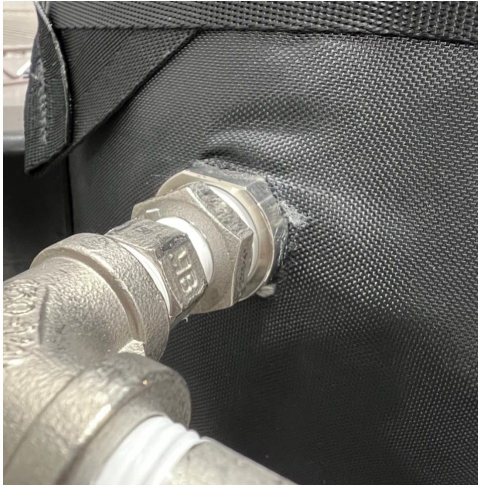
Figure 19: A close-up photo of the hole drilled in the heating jacket
