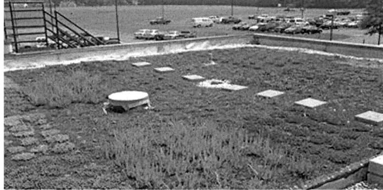
Figure 2-7: Example of a Green Rooftop, Goldsboro, NC
