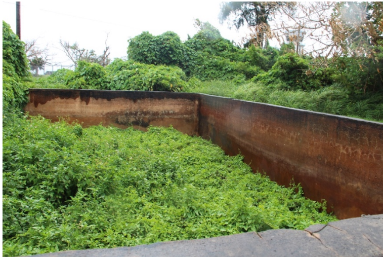
Figure 1: Water holding tank behind power plant facility, Isley Field, Saipan (Photograph by Author)
