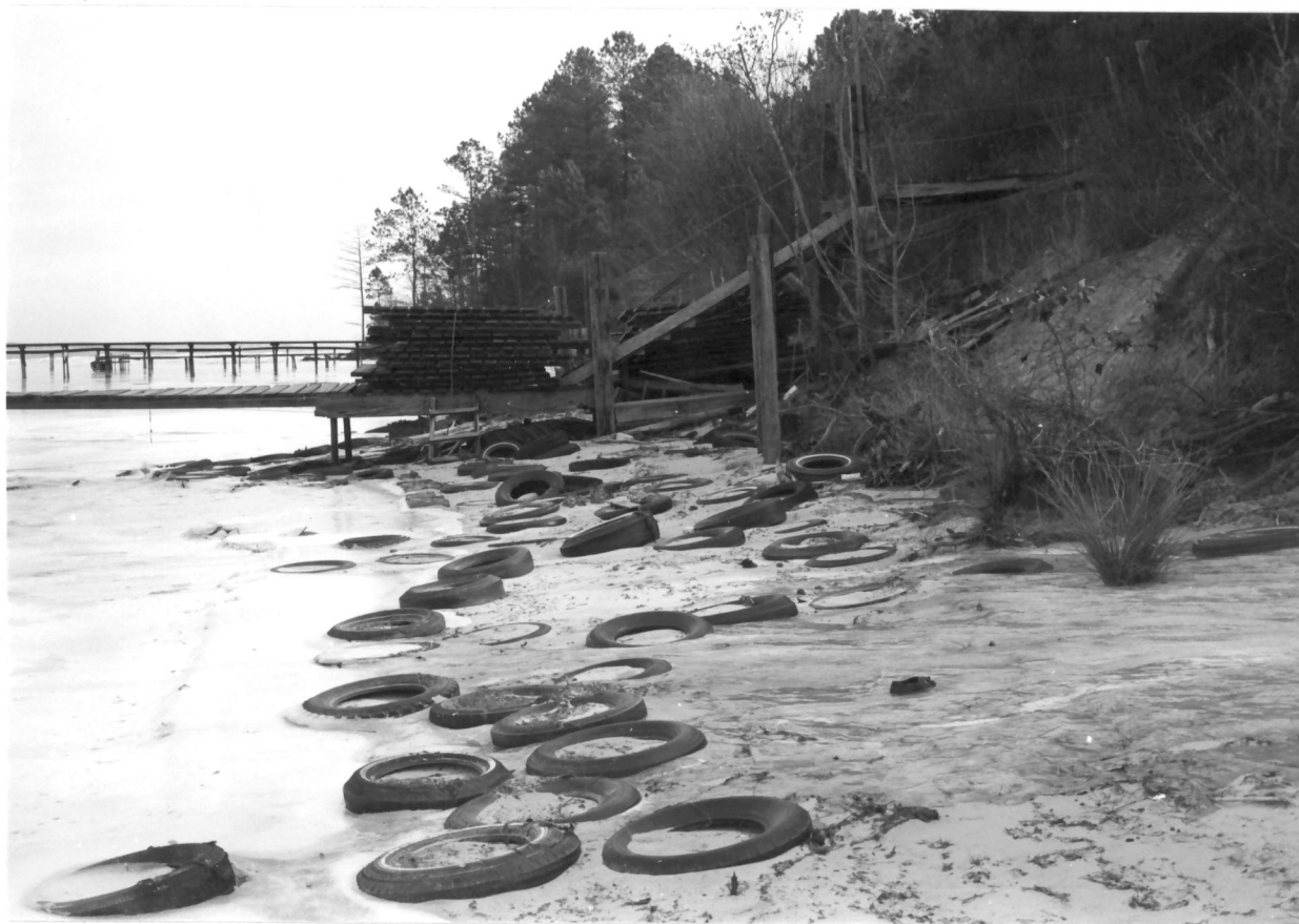
Fig. 17. The use of tires to deter erosion at the base of a Type IV shoreline located on the south shore at Tripp Point.
