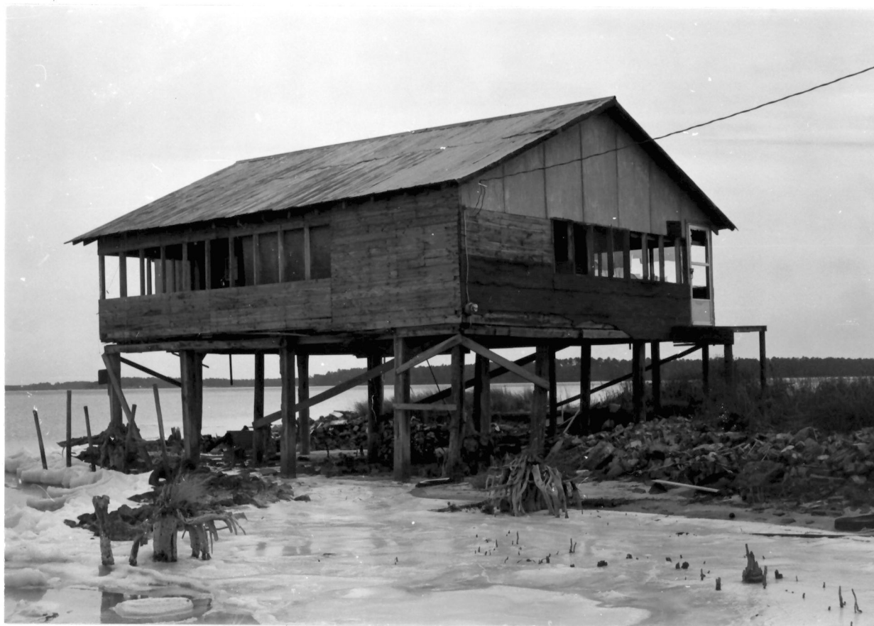
Fig. 19. Deserted house on pilings on southern shore at Hickory Point. Area of very active erosion. Waves are breaking under the house. Attempts have been made to inhibit the erosion by the use of bricks and concrete.
