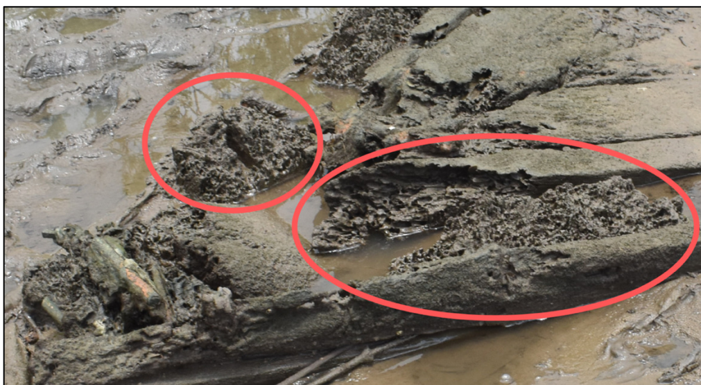
FIGURE 146. Southern end post assembly, note the evidence of degradation via borer insect on portions circled in red (image taken by author 30 June 2024).
