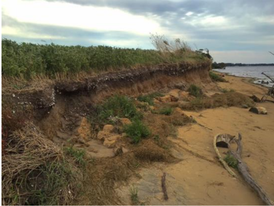
Figure 2.2 Low sediment bank with exposed shell midden. Currituck County. Photo by Lea Abbott
