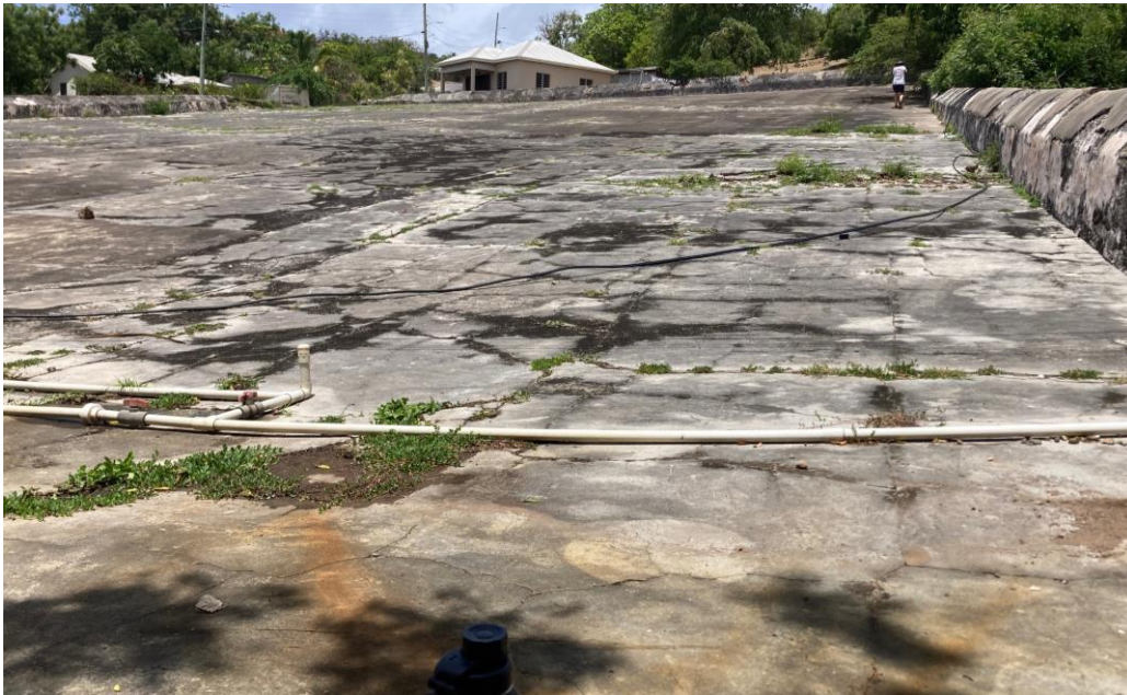
Fig 1.1. The Tank Bay rainwater catchment. (Photo by author, 2023.)
