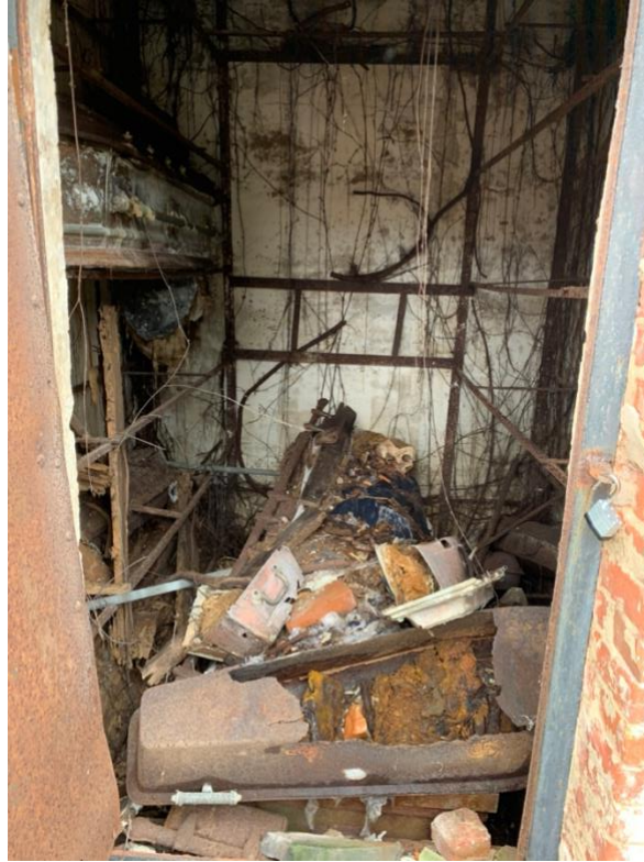
Figure 2: Interior damage of Rhem Family vault as seen from the front door of the vault. F.01 and F.02 are seen laying on the floor across the entrance. Photograph taken by Dr. Megan Perry.
